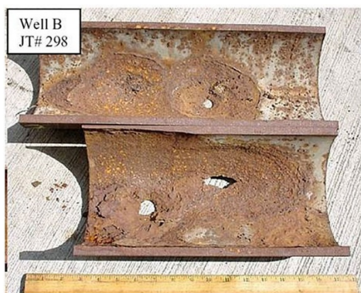
Fig 11: Picture of a well corrosion
